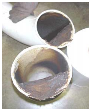
In Only 6 Months The Duct is more than 40% blocked.
