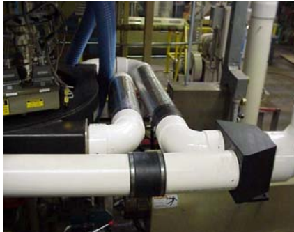
Excellent Ducting Installation
