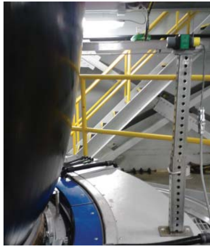
DRJ recently commissioned an IBC Controller, capable of controlling Geo film production as well as Ag film production. Note the newly featured Geo film sensors mounted on the air ring
